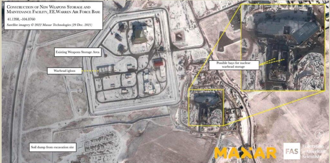
Figure 2: A new underground nuclear weapons storage facility is under construction at F.E. Warren AFB for storage of W78 and W87 warheads for Minuteman III ICBMs. Image: © 2022 Maxar Technologies.
