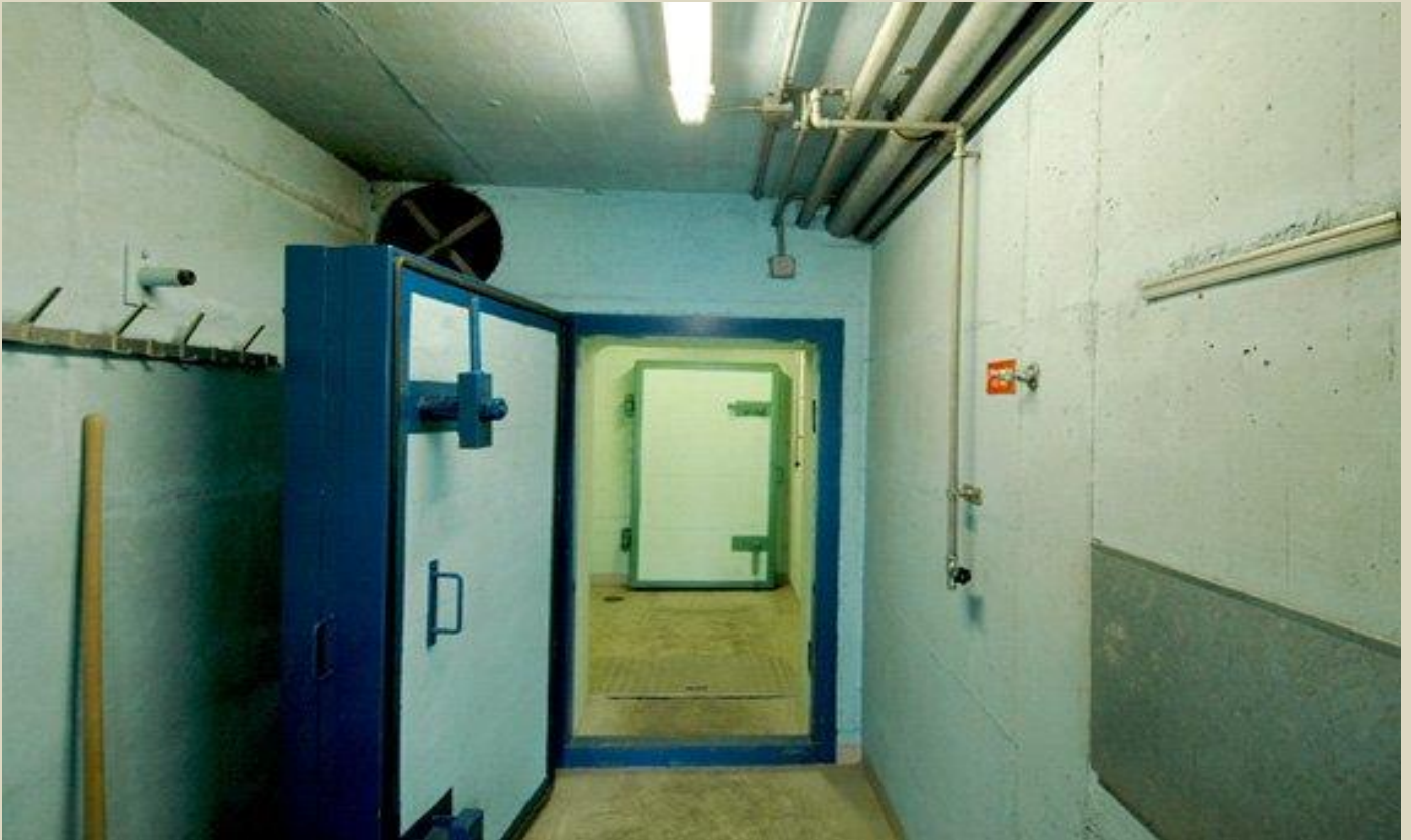
A thick, reinforced steel door leads to Switzerland's largest communal shelter. Photo by Unterirdisch Ueberleben
